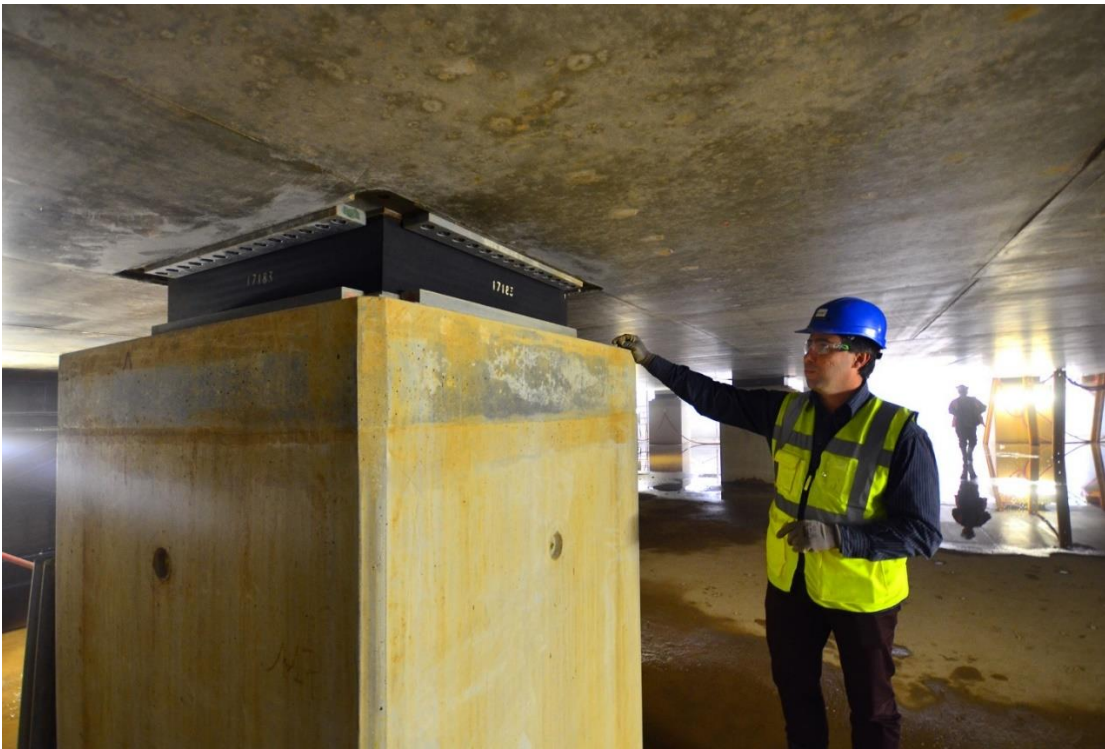
Figure 15 Pedestal, isolator and basemat for ITER showing construction joint at the top of the pedestal. Credit: @ITER Organization
