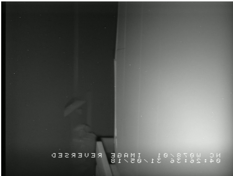
Figure 8: Peripheral Wall Inspection W078/01, Layer 10, Face 3, Brick 1: corner crack.
