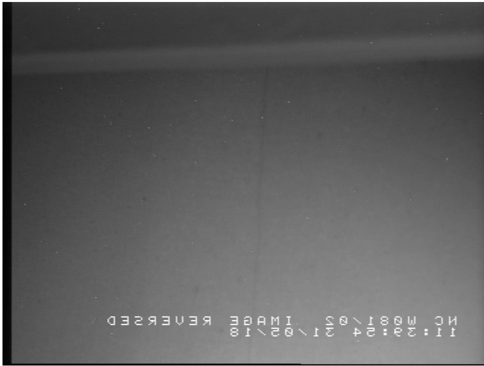
Figure 7: Peripheral Wall Inspection W081/02 – Layer 1, Face 4, Brick 6: linear crack.
