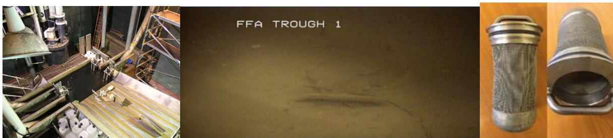
Photograph 7 – Image of Flask Filling Trough area, sludge in Trough & example of Filters currently requiring of debris removal
