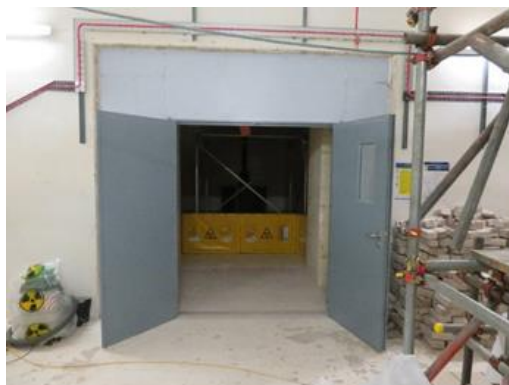
Photograph 8 – Image of the installed C2/C3 (radiological control) doors for access into East Mezzanine room.
